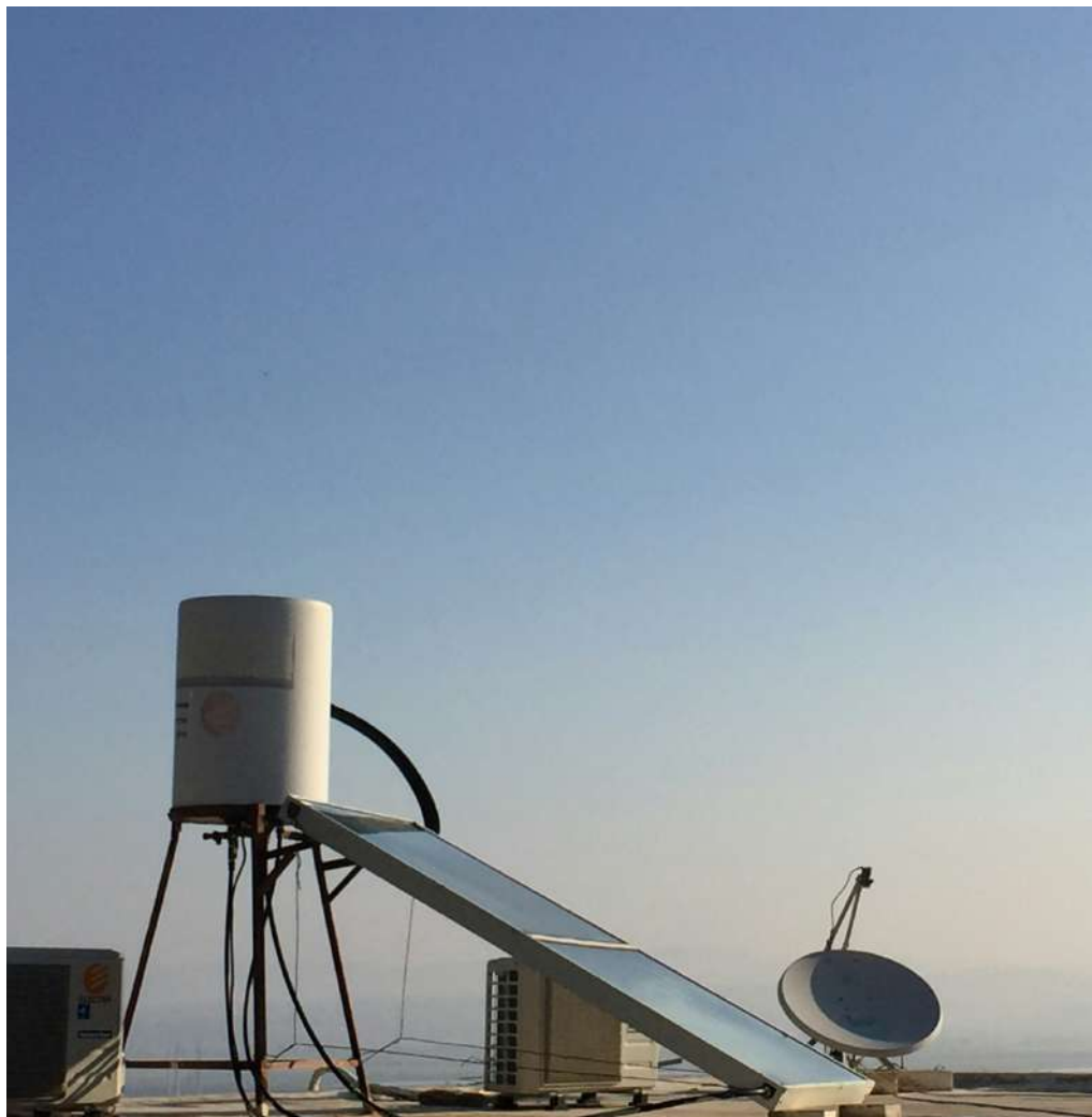
SOLAR BOILER 150L OR HEAT PUMP 150L
